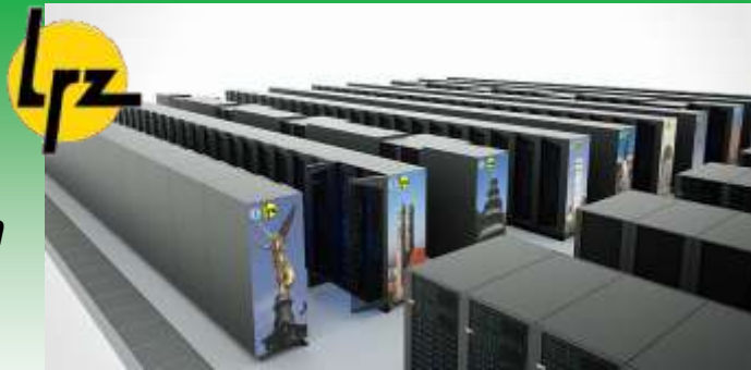
LRZ SuperMUC Europe-wide research cluster 9,587 servers, direct-water cooled
